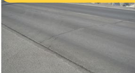
Crack seal and chip seal needed
