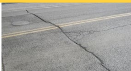
Pavement overlay needed
