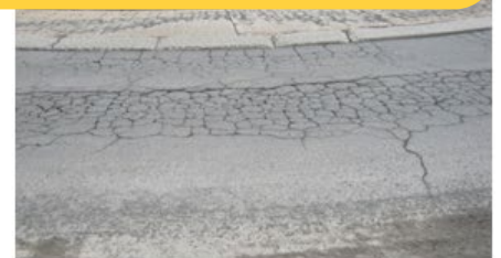
Pavement inlay needed
